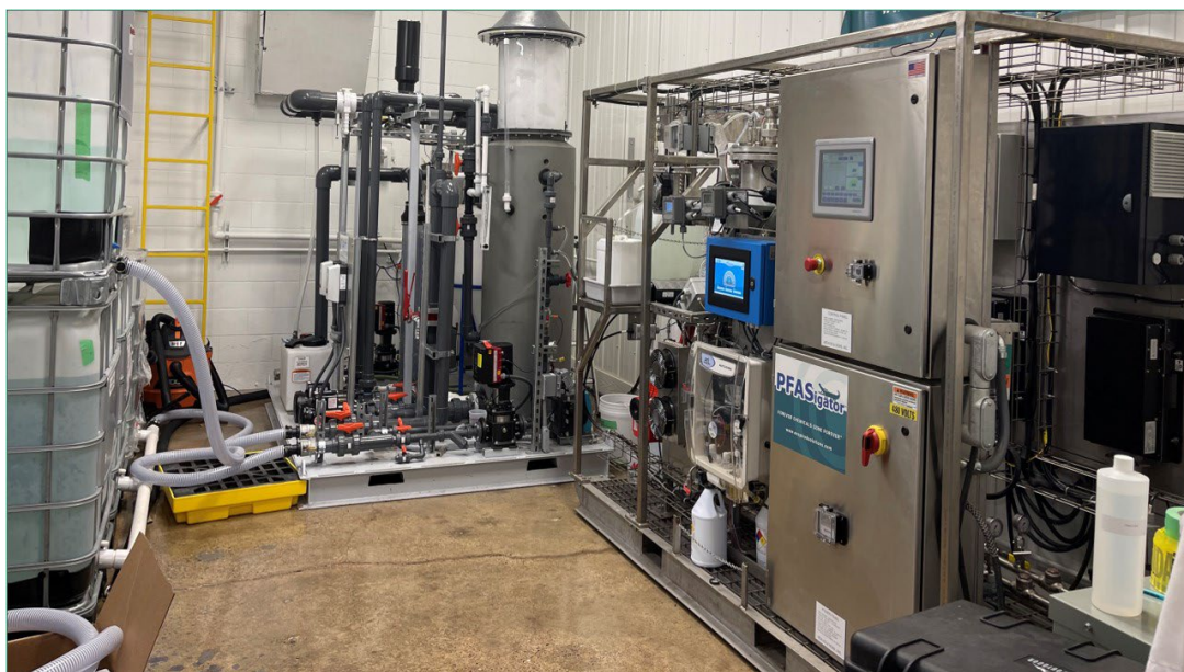
Figure A1-4-1 — PFASigator pilot demonstration, November 2023. Pilot-scale treatment plant including totes of contaminated groundwater (left), the foam fractionation unit (center back, provided and operated by ECT2) and PFASigator (right).
