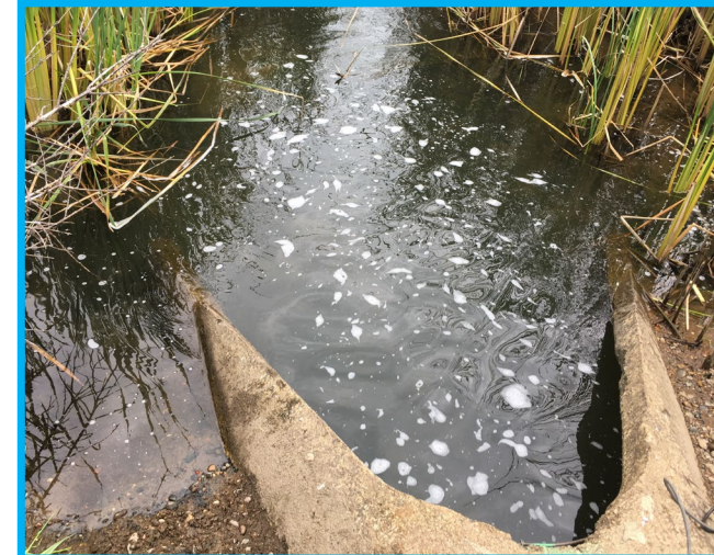
High flowing water exiting a culvert created significant turbulence, resulting in foam bubbles observed downstream of Horseshoe Lake.
